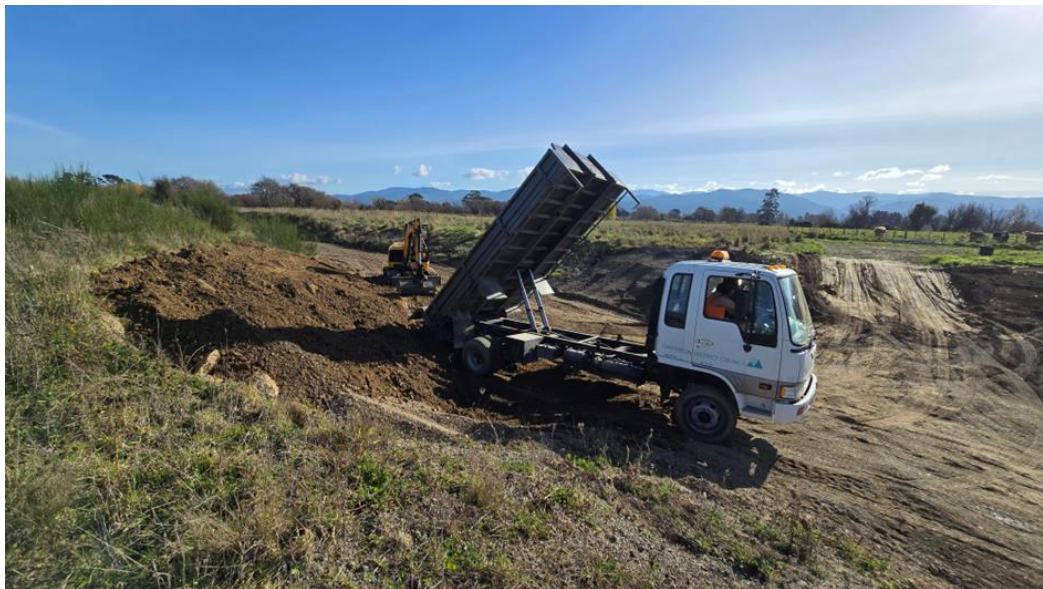
Figure 2 - Image showing CDC maintenance works progressing to restore the eroded bank, remove or manage silt build-up where required, and maintain the function of the ephemeral channel.
