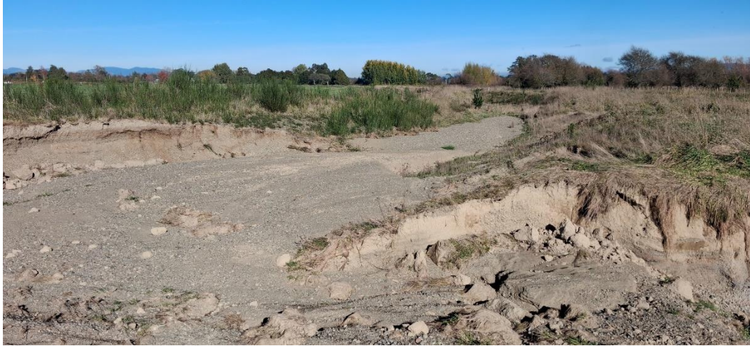
Figure 1 - Image showing the condition of the ephemeral channel at the rear of Te Uru o Tāne Nursery following the April heavy rainfall event, including silt build-up, and localised bank erosion adjacent to the Phase 3 planting area.
