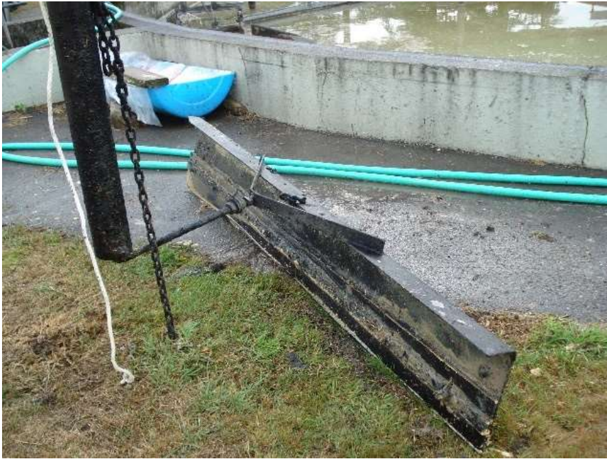
Likely condition of the scrapers with worn rubbers and corroded steel work.
