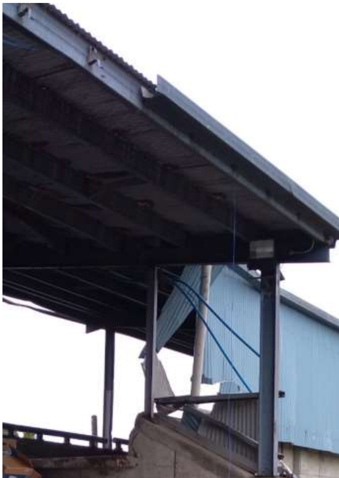
Showing damaged Cladding and missing Spouting.
