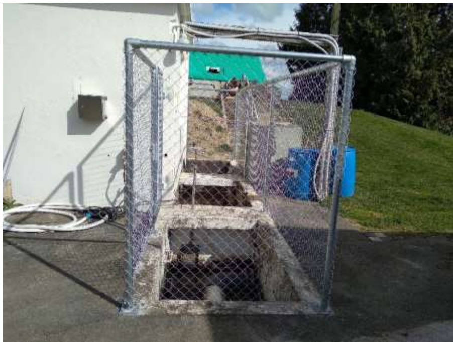
New Fencing and Gate around the Open Channel into the Pump Room.
